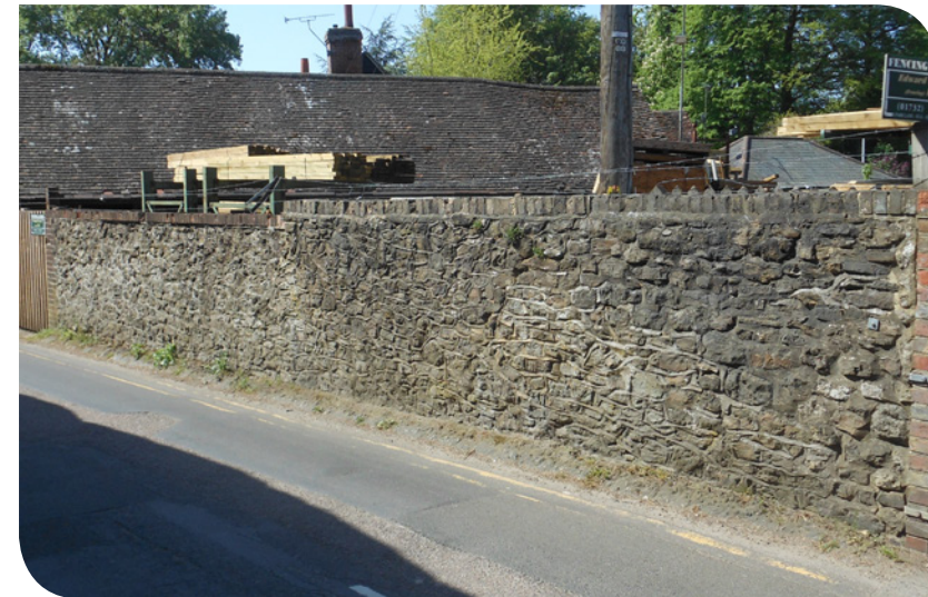
Inappropriate pointing to some ragstone walls
